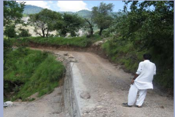
Link road in Gulmera village Talhatta UC under rehabilitation with Community Investment Funds of ERRA
